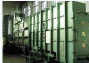
Vacuum tank (vacuum percentage 98.7%; flow discharge 1.0 m 3 /s)
